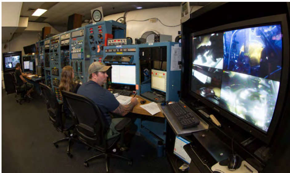
Figure 4. Control room of the NEDU facility (photo courtesy Steven Frink).
